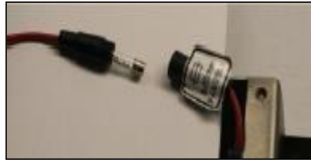
Figure 6 - Battery Backup Fuse
