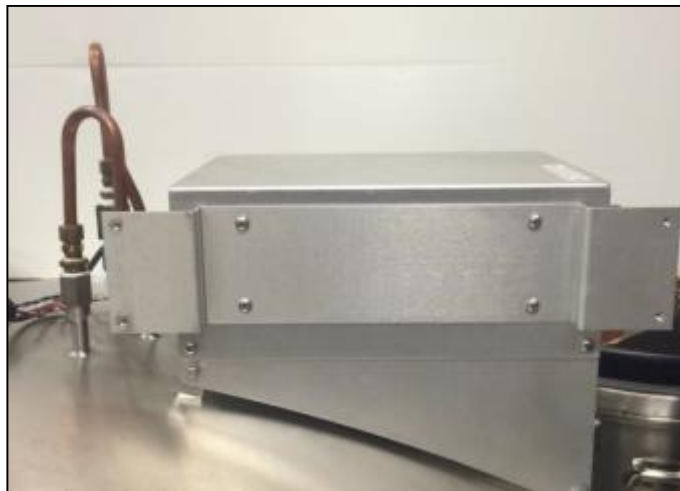
Figure 5 - Vario Battery Backup Bracket Installed
