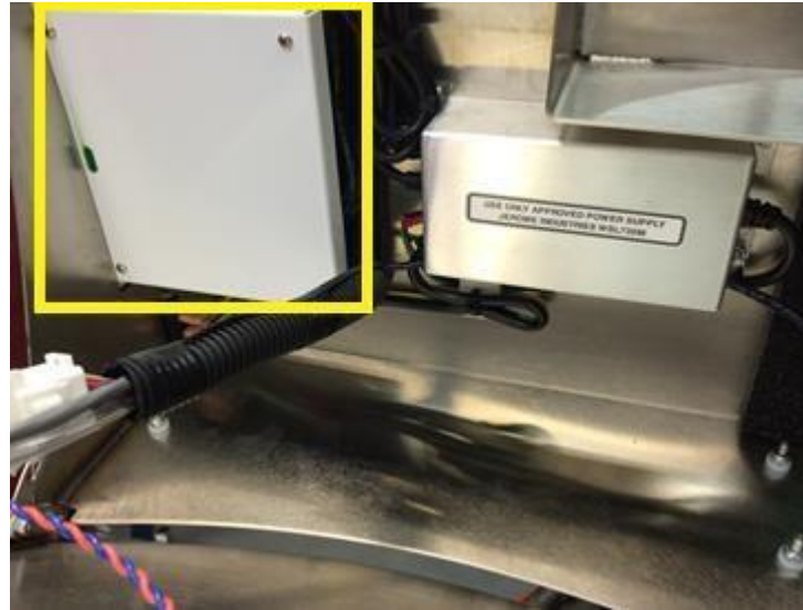
Figure 14 - Back Control Panel
